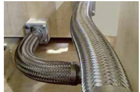
Flexible flow and return hose sections attached to the transformer.
