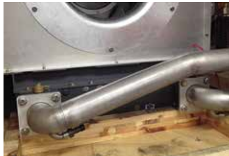
Rigid hose line end attached to the radiator.
